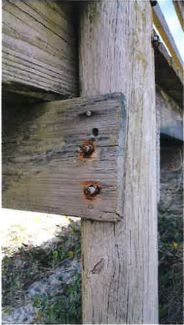
Corroded Bolts and Nuts at Girder
