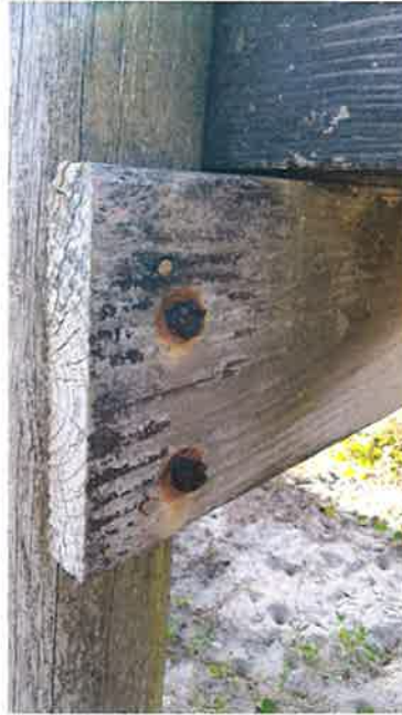
Corroded Bolt Heads at Girder
