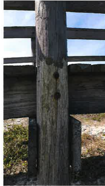
Corroded Bolt Heads at Joist to Piling
