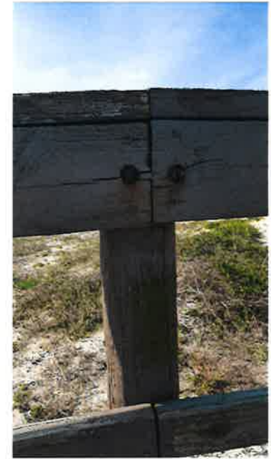
Corroded Bolt Heads at Guardrail to Piling
