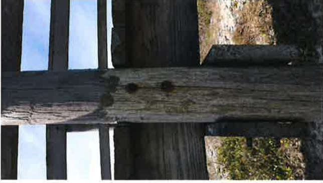
Corroded Bolt Heads at Joist to Piling
