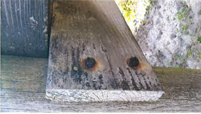
Corroded Bolt Heads at Girder
