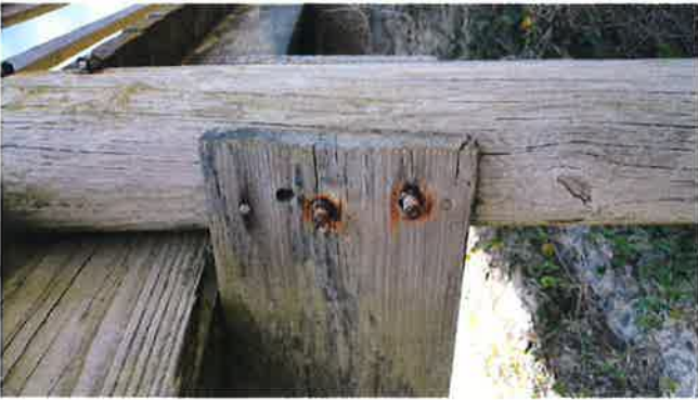
Corroded Bolts and Nuts at Girder
