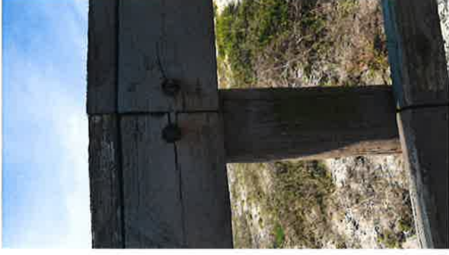
Corroded Bolt Heads at Guardrail to Piling
