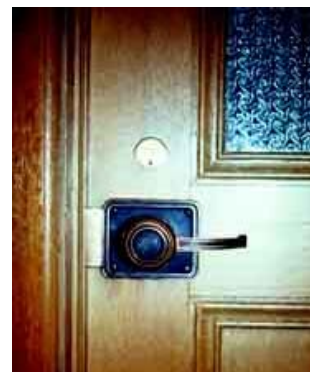
This door handle has been retrofitted to meet ADA requirements. Photo: NPS files.
